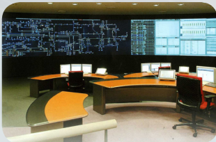
Electric Utility Control Center
