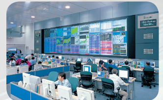
Network & Communication Center
