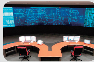
Traffic Control Center
